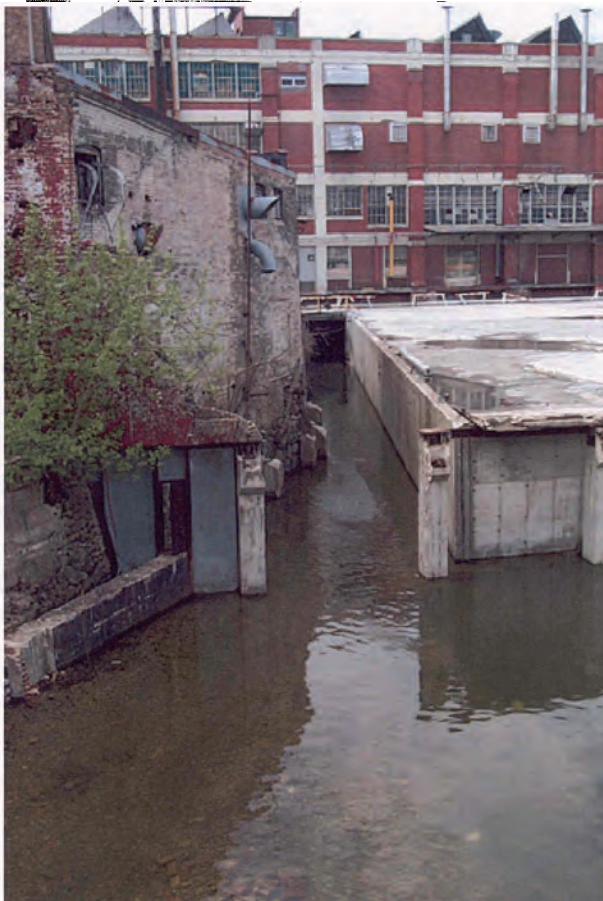
View of existing race looking west as it is diverted under the Uniroyal Plant.
