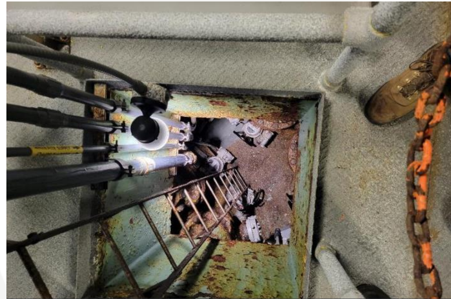
Corrosion in Filter Room
