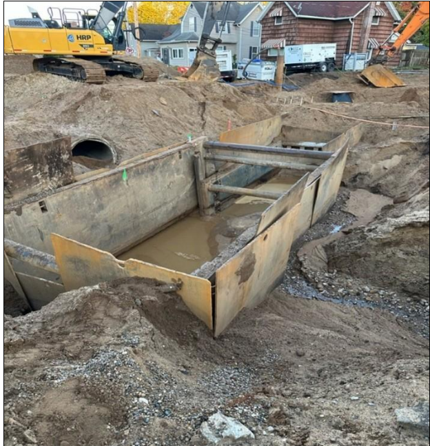
Flooded Trench Box about 48 hours after incident
